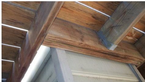
Missing hangers @ beam, joists not doubled
