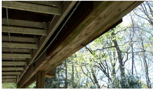
Beam break not supported by post to transfer loading
