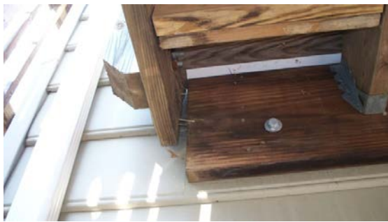
Substandard construction not to current standards
