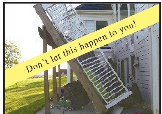
Photo Courtesy of NADRA Member: Simpson Strong-Tie
